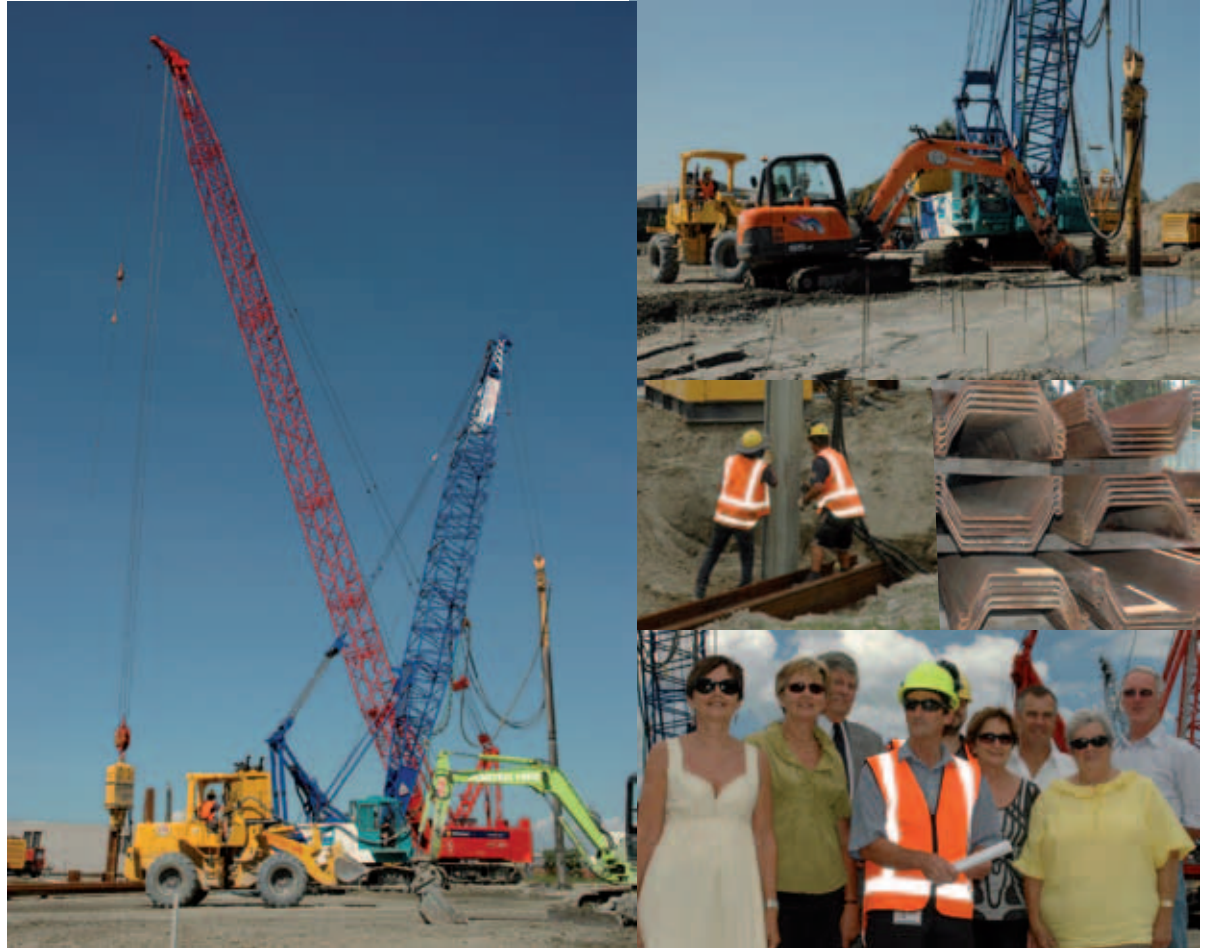
The $40M city wastewater project is the largest infrastructure project undertaken in more than 40 years. Clockwise from left, the dance of machinery; constructing stone columns; sheet piling; and operations committee members with project manager Peter McConnell.
