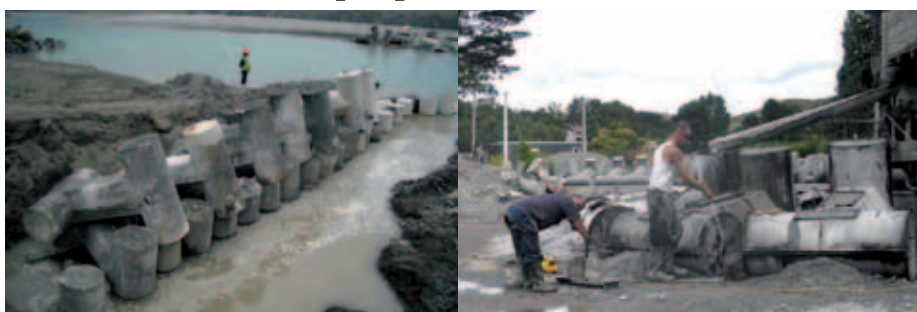
Dolosse in place in the Waiapu River. Ruatoria workers (right) help construct the concrete blocks.
