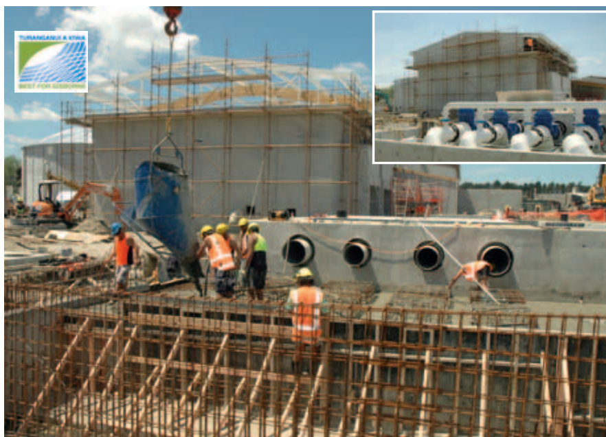
It's progress every day on the Banks Street site. The pipes coming out of the outfall pump station (centre) now go into a central manifold. Treated wastewater will soon be pumped 1.8km to sea. The pre-treatment building (centre back) now has its roof (inset) and the trickling filter tank (back left) is 99% complete.
