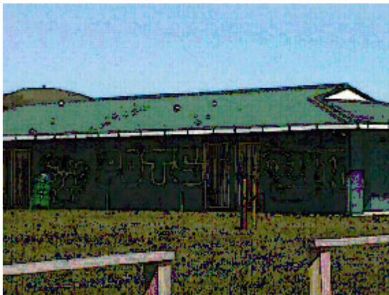
Photo 1 : The ablution block is always covered in graffiti.
