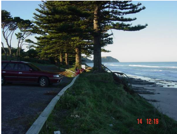
Pines carpark and bank showing erosion and plant pests
