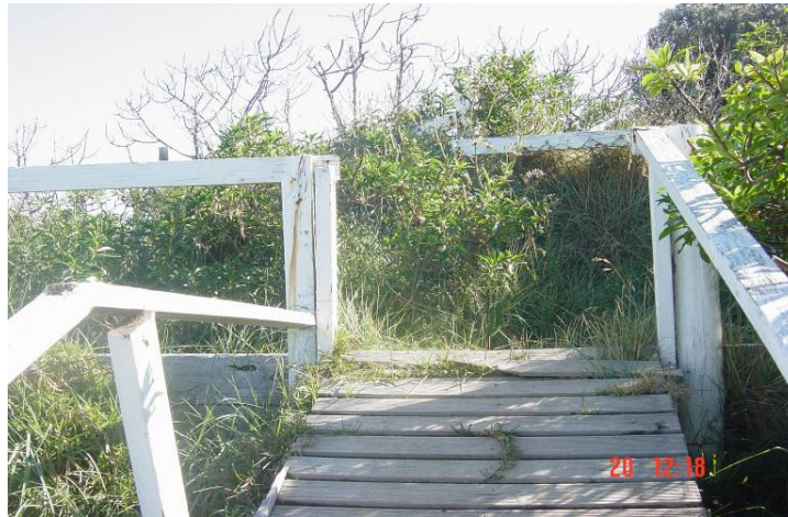
Figure 12: Steep ramp with broken railings showing rot at the top.
