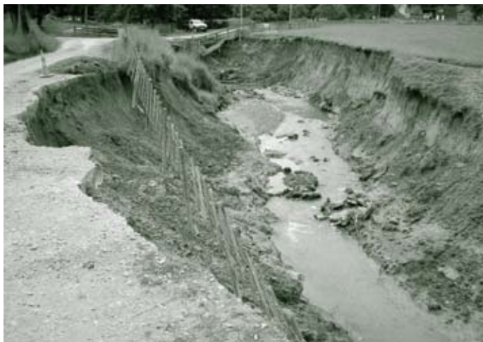
Above: Damage to Pakowhai Road, Muriwai, after the 2005 floods.
